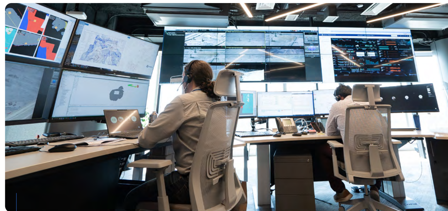
Anglo American has taken another step towards mining in the future with its new Integrated Remote Operation Centre (IROC), which will allow Los Bronces mine to be controlled in real time, and in an integrated way, from a control centre in Santiago, 67 km away from the mine.
