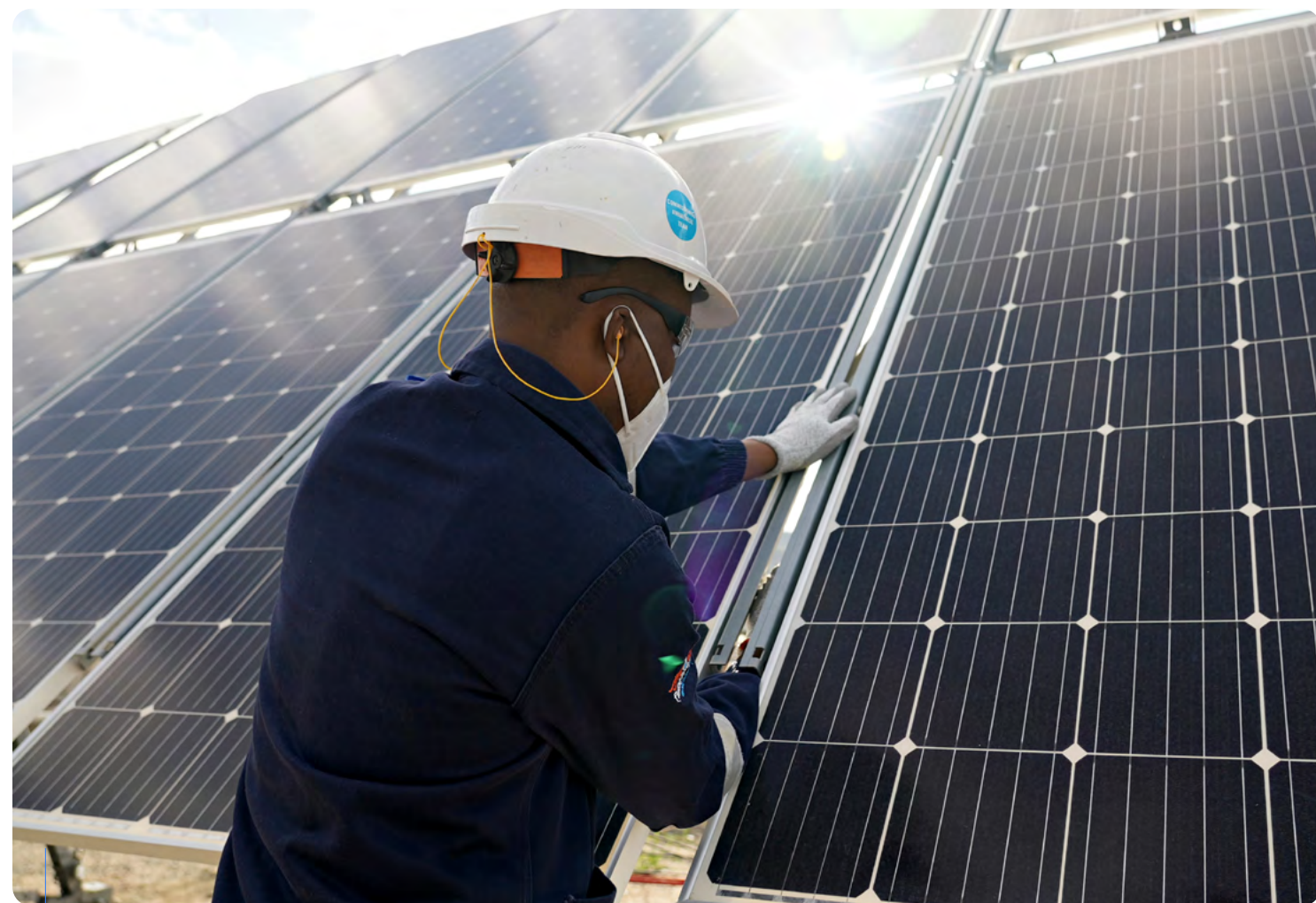
General assistant James Kutumela, assembling photo-voltaic (PV) panels for the solar-powered hydrogen plant under construction at our Mogalakwena PGMs mine.
