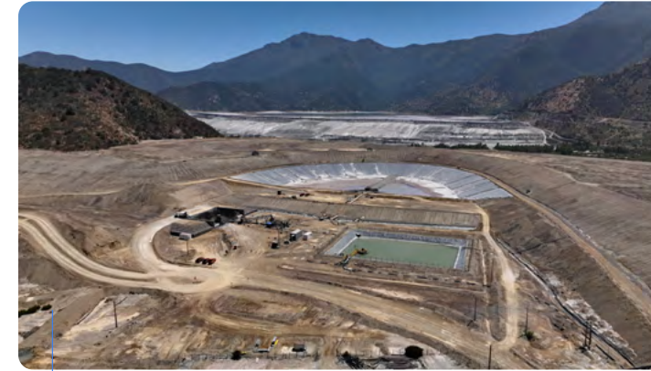
Hydraulic dewatered stacking (HDS) is an emerging technology that allows the safe disposal of mining by-products and accelerates our progress towards the end of wet tailings storage. Featured is the demonstration plant at our El Soldado copper operation in Chile, where HDS technology is being trialled on a large scale.
