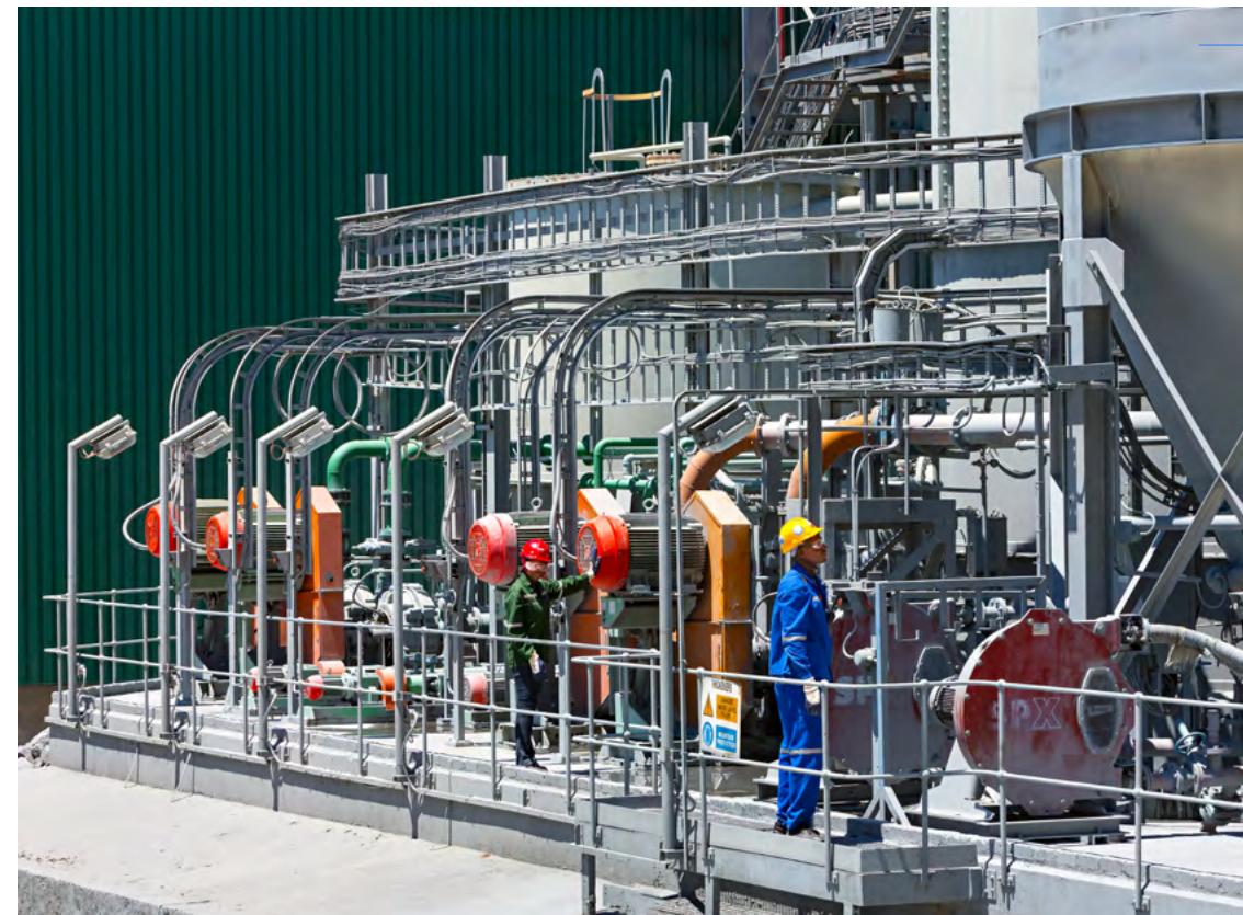
Inside the concentrator plant at PGMs' Unki mine in Zimbabwe. Unki is the first mine in the world to publicly commit to a third-party audit to determine its performance against the Initiative for Responsible Mining Assurance (IRMA).
